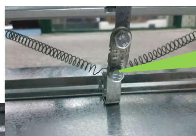
Fire damper only using fuse 74 degree
